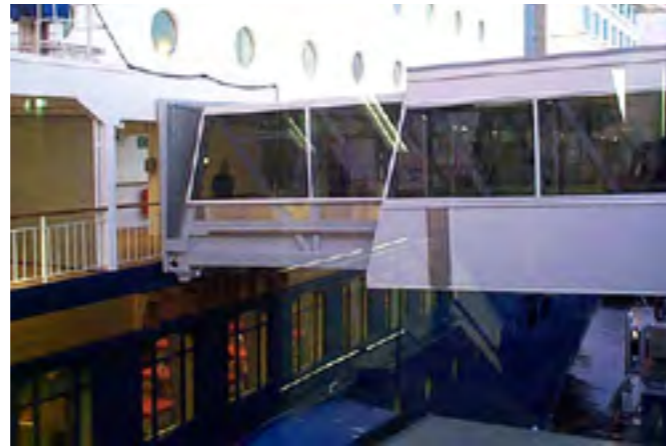
Large movements of the ship may cause damage to passenger gangways, ramps, linkspans and harbour structures.
