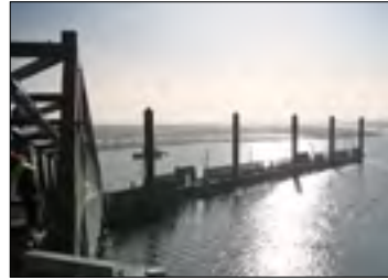
2013 Floating pontoon terminal Eight service vessels can transfer crew and supplies to/from offshore windfarms. Port of Mostyn, United Kingdom BAM Nuttall
