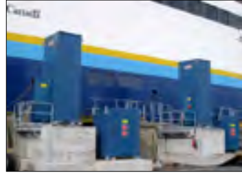
2010 & 2009 Four MOOREX® 35T ashore mooring systems Port of Basques and North Sydney, Canada Marine Atlantic
